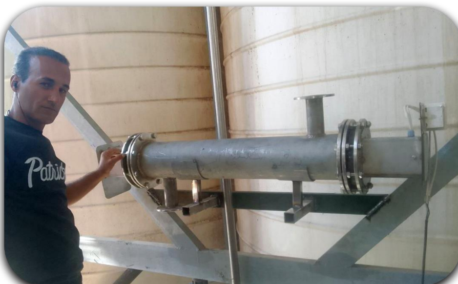
Ozone Gas Removal from the Outlet of Inline (UV-based) Treatment Package
