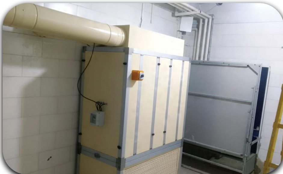
Air Purification System for the Treasury Department of Post Bank, Qazvin
