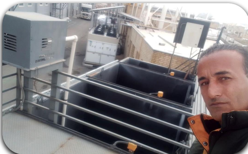
Wastewater Treatment Package for Avrand Pishro Industrial Complex
